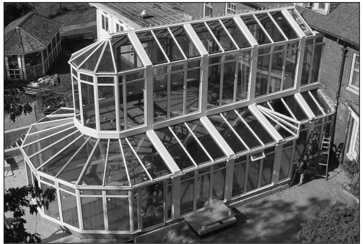
Workers put the finishing touches on Sea View's new conservatory. The glass ceilings and walls will provide a bright and cheery setting year round.
